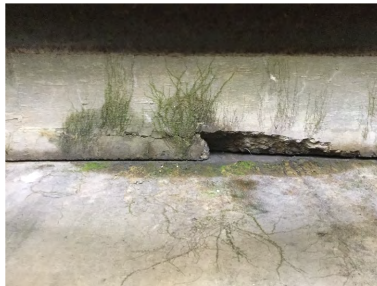
Panel damage at right bank
