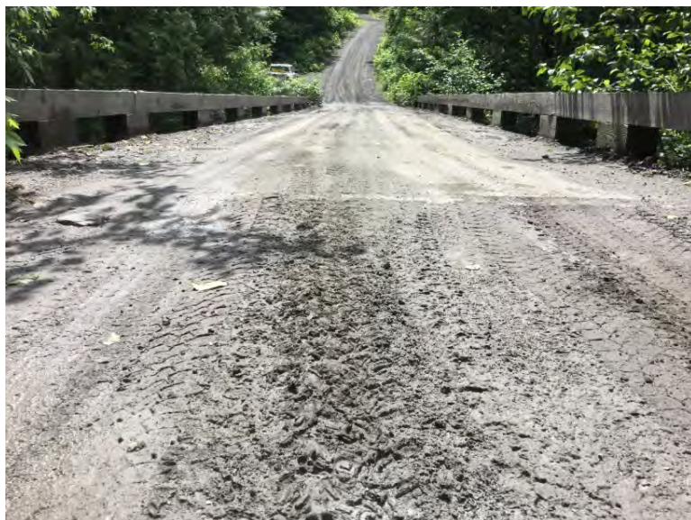
Could use additional fill at right approach
