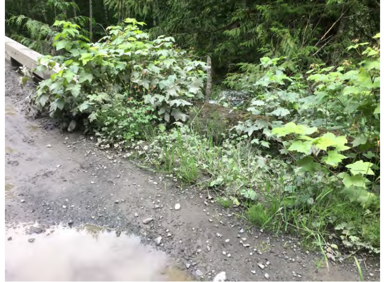
Upstream left bank fender log has fallen off road
