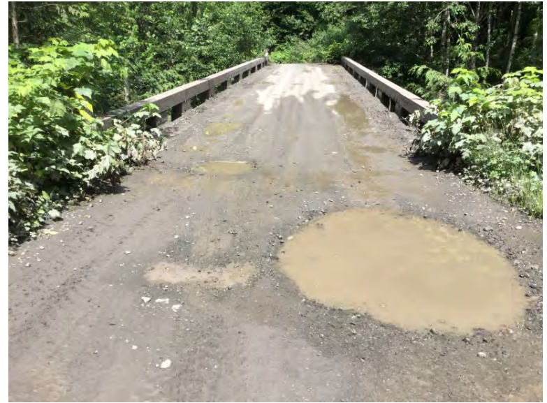
Potholes at approaches
